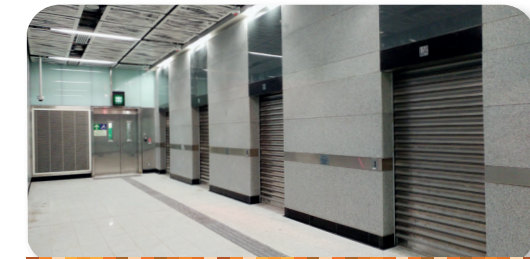
The lifts will stop serving the lift lobby. Fire shutters at lift doors in the lift lobby will stop the spread of fire and smoke into the lift shaft, so that the lifts can be in service for passengers waiting in the Refuge Area.
