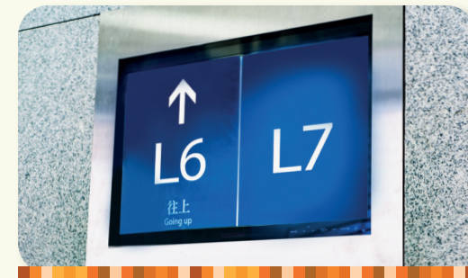
Monitors show the position of the lift and its direction.
