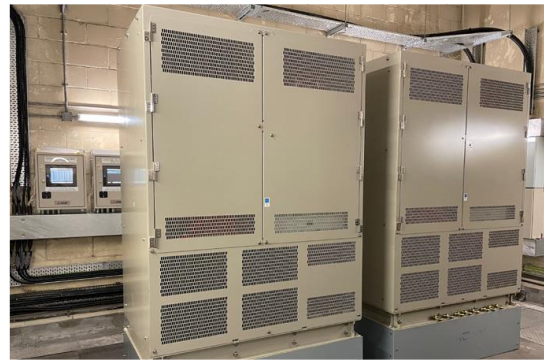
Energy Saving Inverter systems at station
