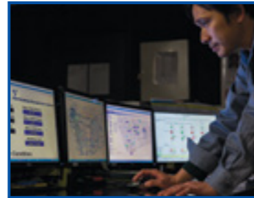
Control Centre Elements shopping mall in Hong Kong uses state-of-the-art control systems to keep the mall at a comfortable and energy-efficient 25°C year round.
