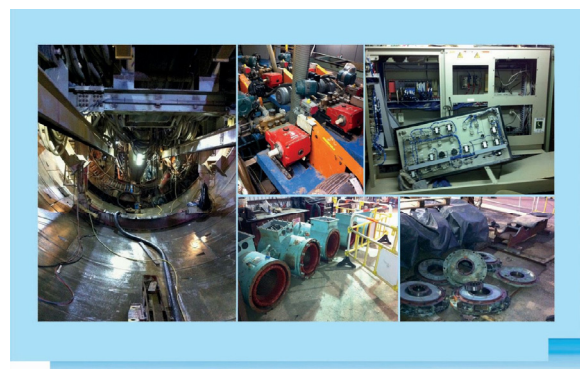
Damaged TBM at contract 823A
