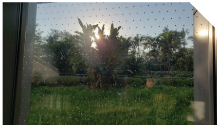
(Upper) A set of stickers along the interchange walkway with graphics resembling birds (Lower) Installation of anti-bird collision window films on over 100 window facades in Mei Foo Station
