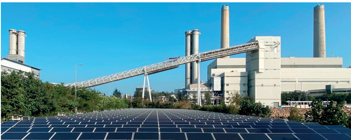
The solar energy generation system installed by HK Electric at its Lamna Power Station
