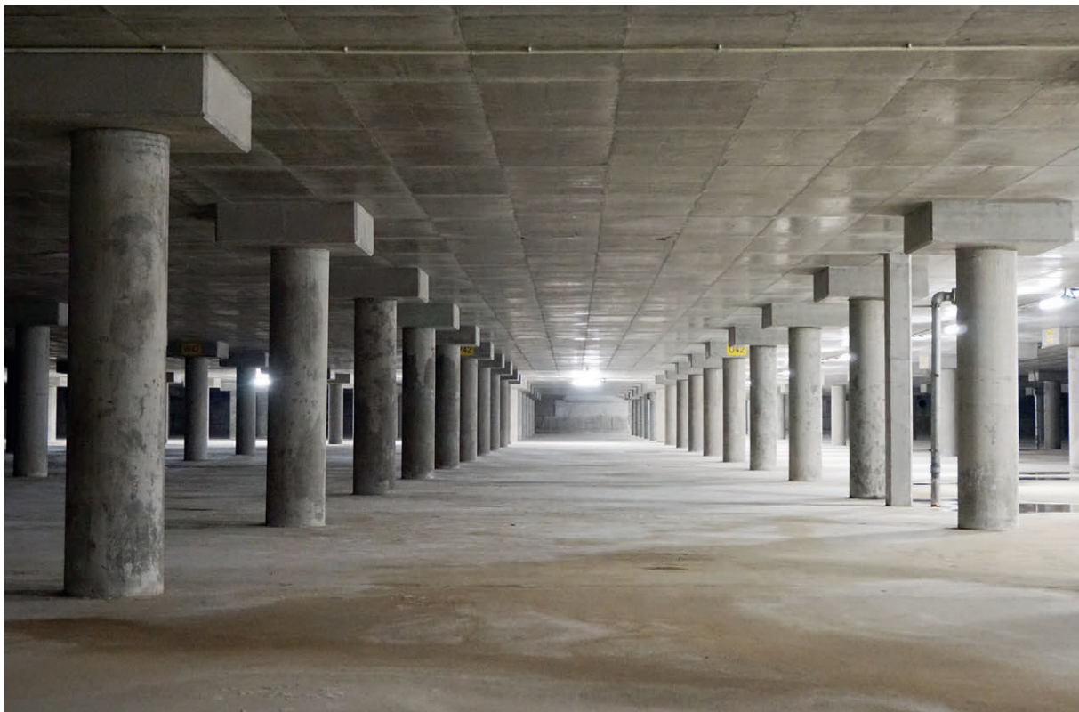
Happy Valley Underground Stormwater Storage Scheme: The stormwater storage tank has a capacity of 60 000 m 3 , which is equivalent to 24 standard swimming pools. It greatly reduces the flood risk to the low-lying areas of Wan Chai and Happy Valley
