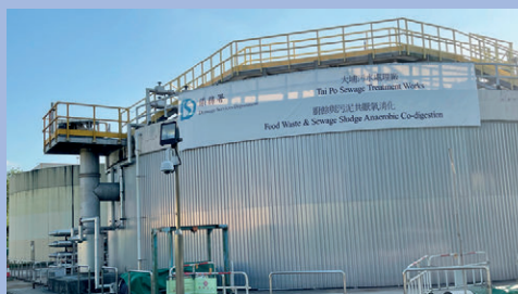
Facility for food waste/sewage sludge anaerobic co-digestion at Tai Po STW
