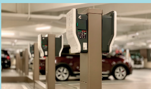
EV charging facilities at the car park of the residential project Grand Central
